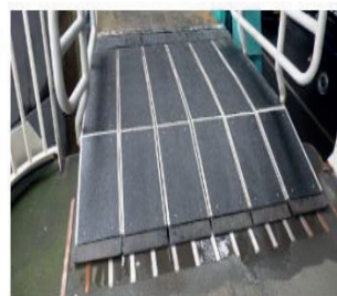
WALKWAY AND RAMP SAFETY
